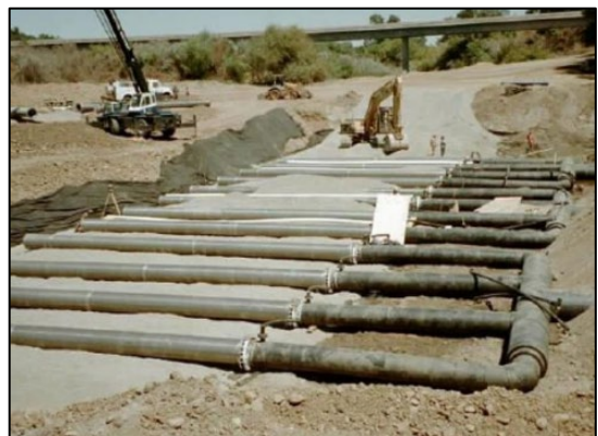
Turlock Irrigation District's subsurface diversion system during construction before being covered by feet of gravel. This system diverts water from beneath the Tuolumne River without harming salmon and steelhead.
